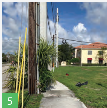
5 Maintain overgrown landscaping
