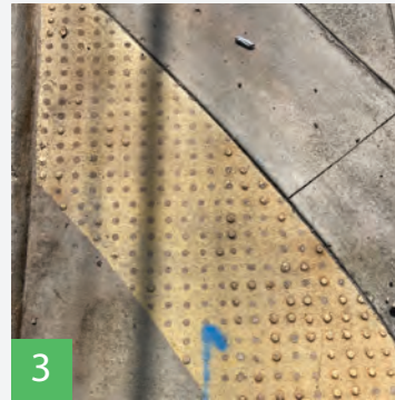
3 Replace worn detectable warnings
