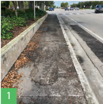
1 Fix uneven asphalt sidewalk
